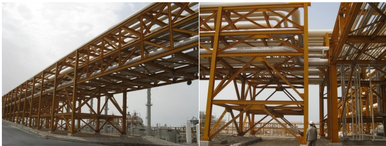
Picture1: Picture of pipe and pipe rack
