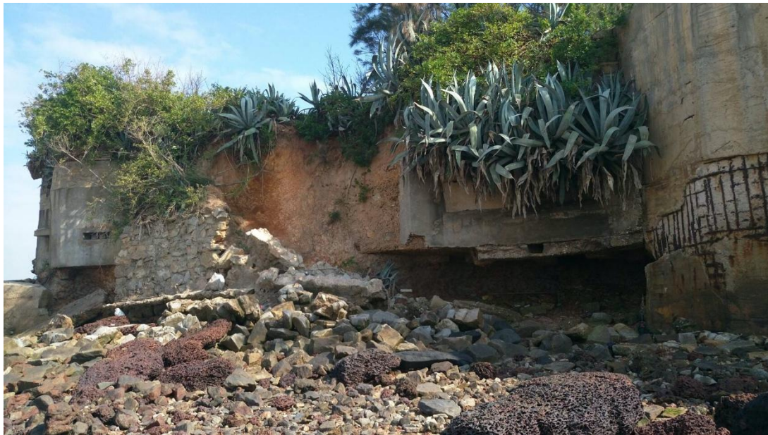
Figure 8. Foundation of Coast Fortress Has Been Washed Away (Hsu, C. H, 2016)
