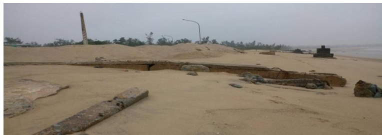
Figure 9. The Bottom of Bollard for Navy Landing Boat's Supply Operation is exposed and Street Lamp Pole is collapsed (Hsu, C. H. ,2016)
